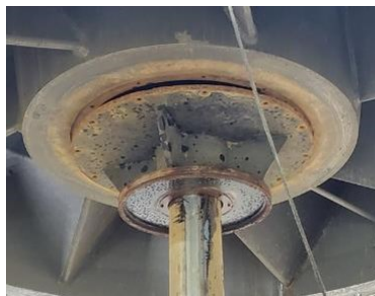
Lower diffuser bearing housing with missing bolts
